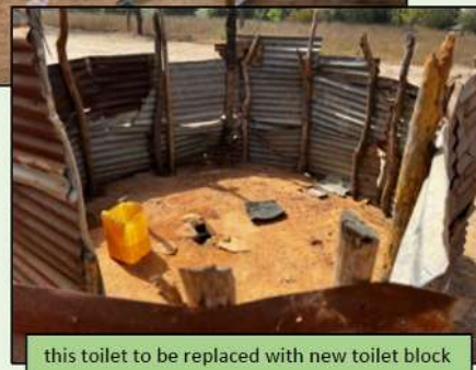
this toilet to be replaced with new toilet block
